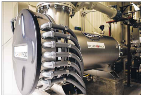
A treatment system, designed to remove contaminant 1, 4-dioxane from groundwater, at a pump station in Central Islip.
